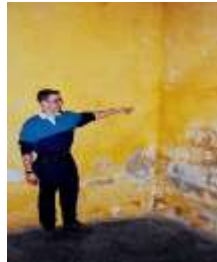
Severe wall water/ceiling damage
